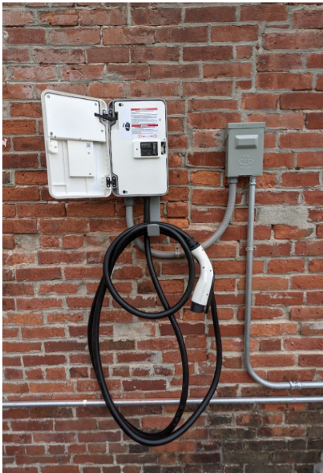
Incorrect installation. External disconnect needs to be removed
